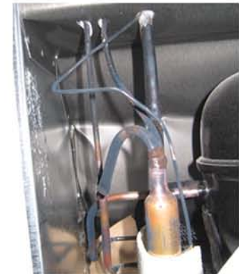
An example of corroded copper piping, as by the contaminated drywall.
